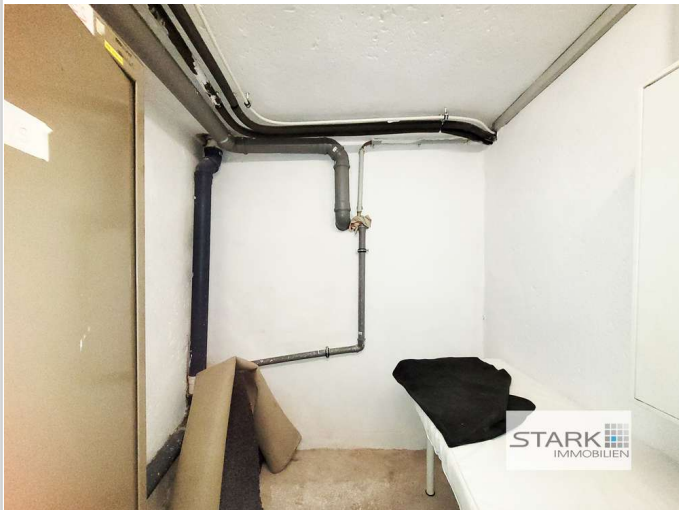
Installation Wasser i O
