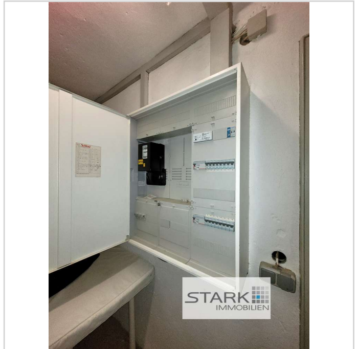
Installation Elektro i O
