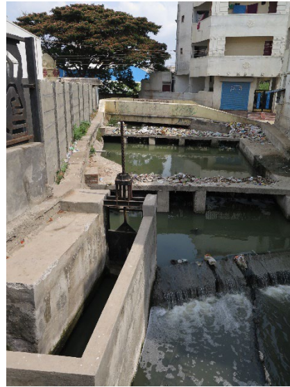
Figure 2: Inlet to Wastewater Treatment Plant at Selvachintamani Lake in April 2022. Source: AQUA-Hub Project Team (Liehr)
