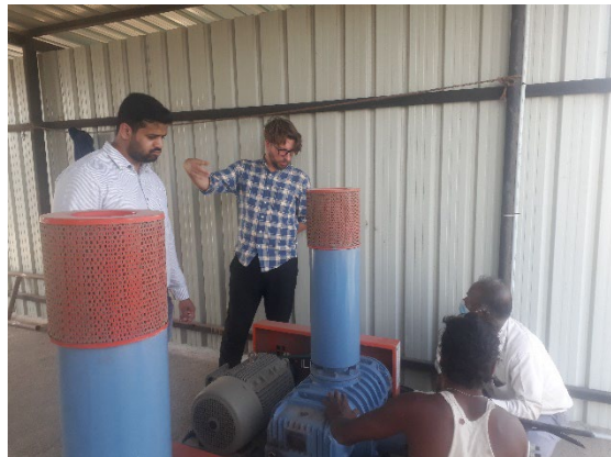
Figure 4: AQUA-Hub Team at Selvachintamani Lake Wastewater Treatment Plant in September 2022. Source: AQUA-Hub Project Team (Prakash)
