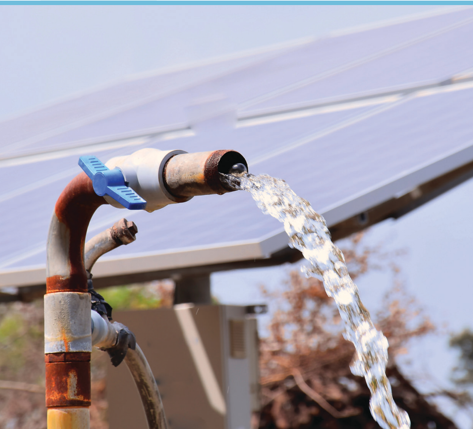
Equipment for a solar-based irrigation project.
