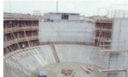
12,000 m 3 seasonal storage, Friedrichshafen, Germany
