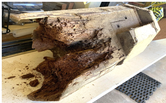
Eight-sided column wood rot
