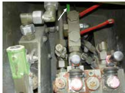
Figur 23 - Blockhahn am Hydrauliktank
