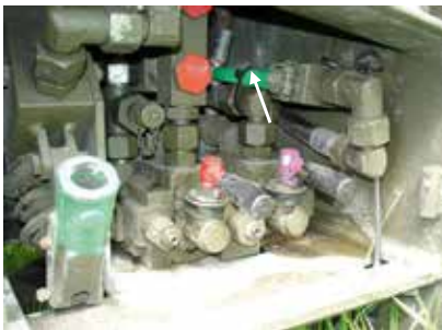
Figur 22 - Blockhahn am Hydrauliktank
